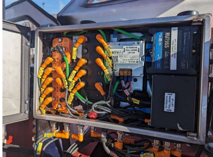
Figure 2 109086 Main Enclosure Assembly Inside View
