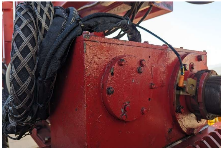
Figure 12 Cables ran from head to mast bulkhead
