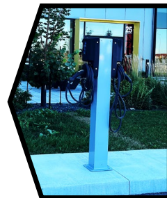
Electric Vehicle Charging Station
