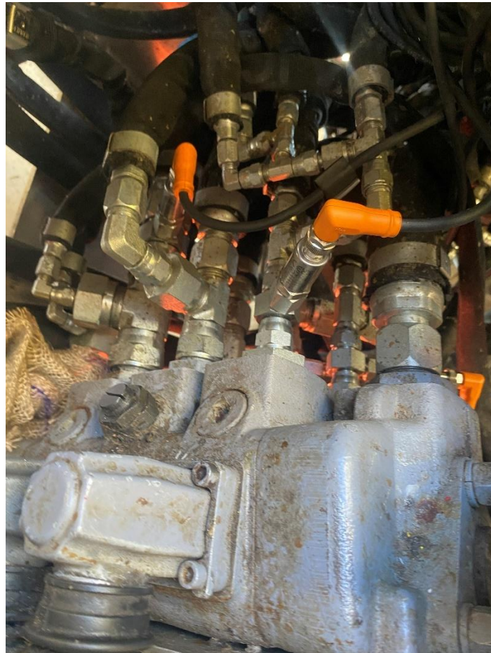
Figure 9 Closer View of Holdback, Pulldown, Rotation Pressure, Wireline Sensor Locations
